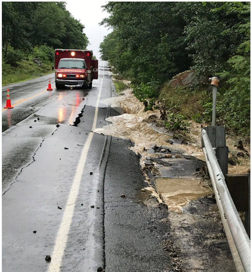
This picture shows ME-129 in South Bristol where intense rainfall in July 2020 caused undermining of the road and washing-out of the ditch. National Weather Service reported as much as 5 inches of rain in the belt between Waldoboro and Waterville and a gage near US-1 in Newcastle reported nearly 3 inches in 24 hours between July 14th and 15th, 2020. Climate scientists generally agree that we can expect more frequent, more intense storms under future elevated greenhouse gas scenarios.
